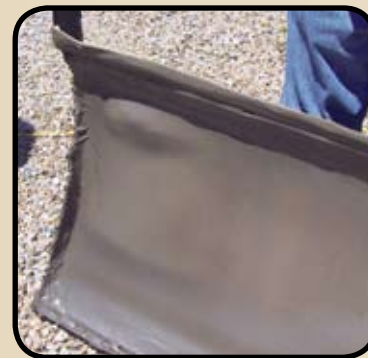
Inside: No Penetration
